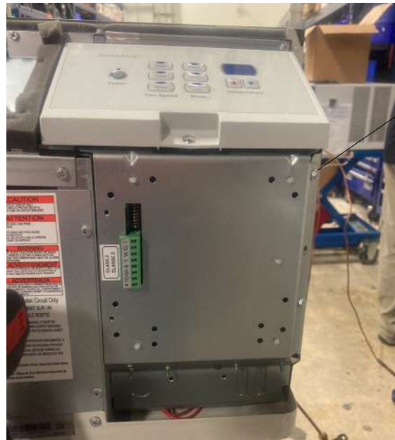
Figure 704 (Open Electrical Box)
