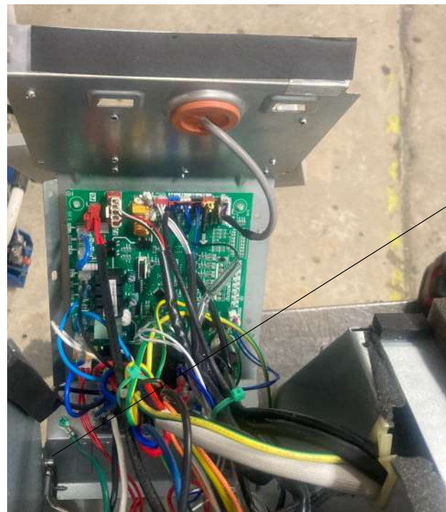
Figure 705 (Open Electrical Box)
